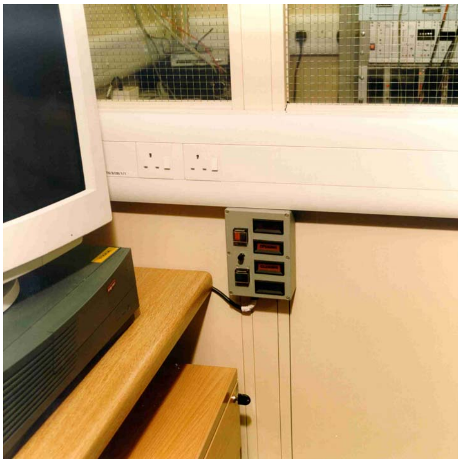
Figure 2.8: The shutter controls in the TOSCA cabin.
